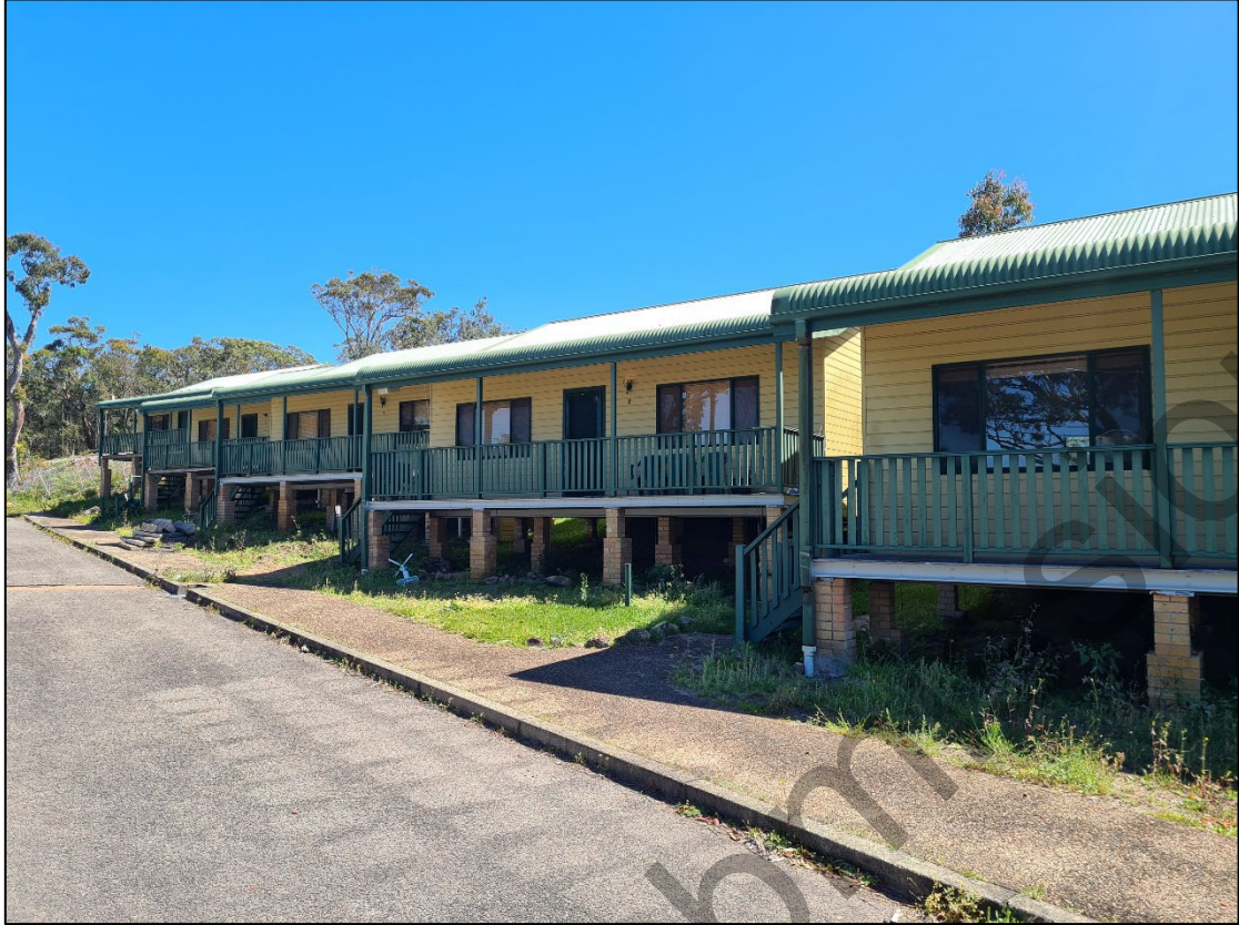
Above: Current dilapidated dwellings located in the southwest of the site.
